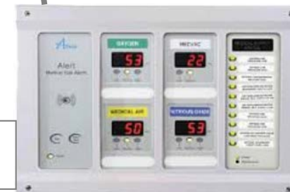
Master Alarm Board
